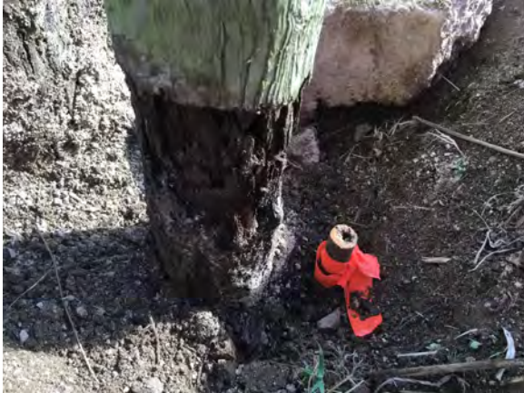
Photo Orientation & Description: Pipe at Q25
